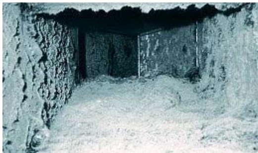
Dirty Air Duct
